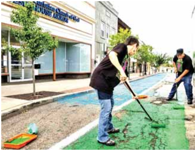
Fran and John Thoricht use washable paint to create temporary extended sidewalk areas for people to congregate.
