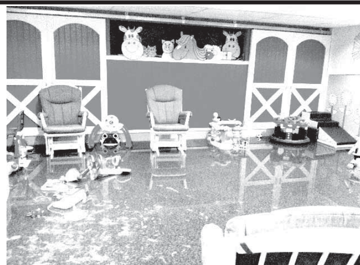
Flooded Basement at First Glance
